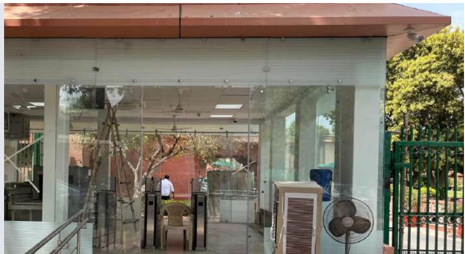
Security gate at the high security zone from gate C of the Supreme Court premises under renovation during summer vacation
