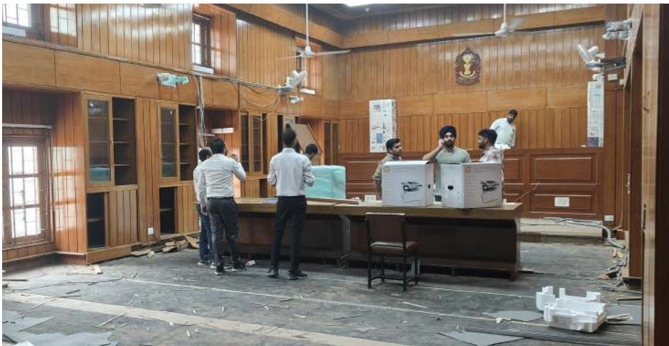
Courtroom no 6 among other courtrooms including 7, 8, and 9 being renovated to make them futuristic and technologically advanced during vacation
